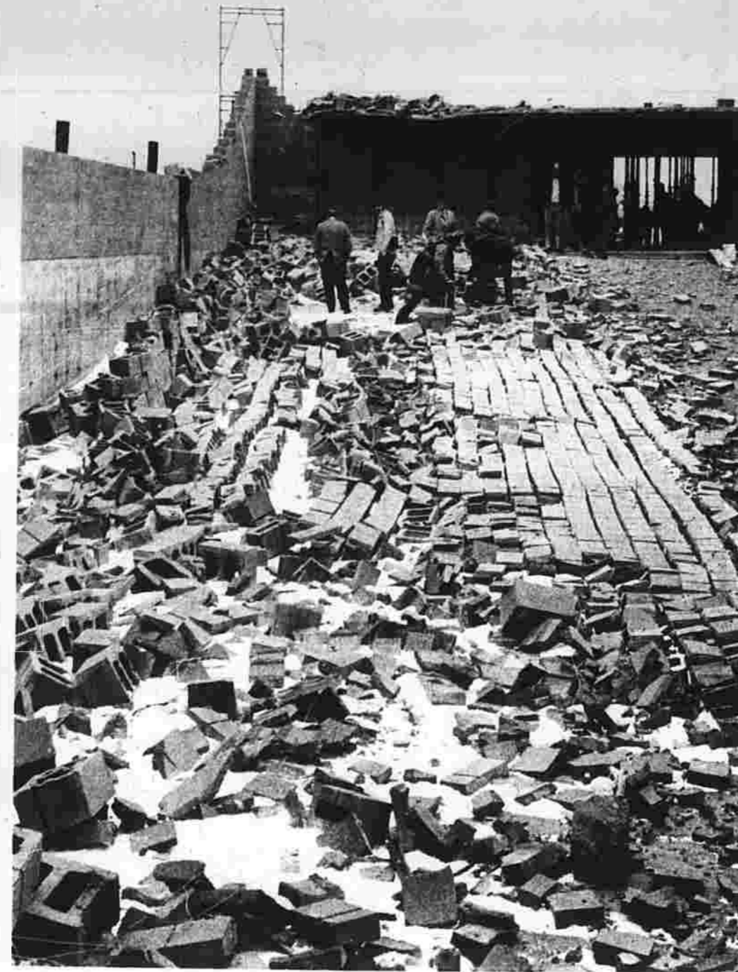
This was the scene last April at East Hartford's Showcase Cinema after a strong wind blew over a wall that was under construction. One worker was killed. (Herald photo by Pinto)
